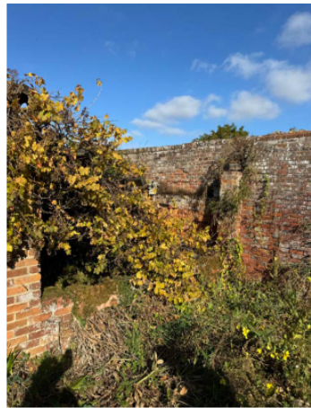
4. View of Loggia from south east end showing timber roof collapse and excessive vine growth
