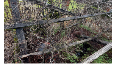
5. View of Loggia from above showing timber roof collapse
