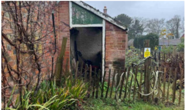
2. South-eastern entrance door to potting shed - timber door frame suffers rot
