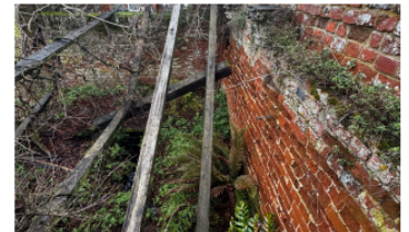
7. View of Loggia showing collapsed timber structure from above
