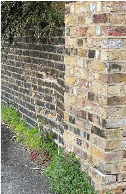
Damaged existing brick wall. Visible cracking to newer brick pier.
