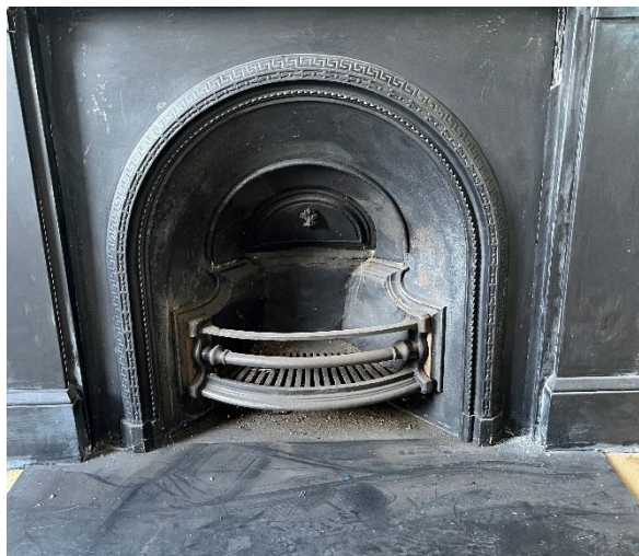
Minor damage where insert abuts the surround.
