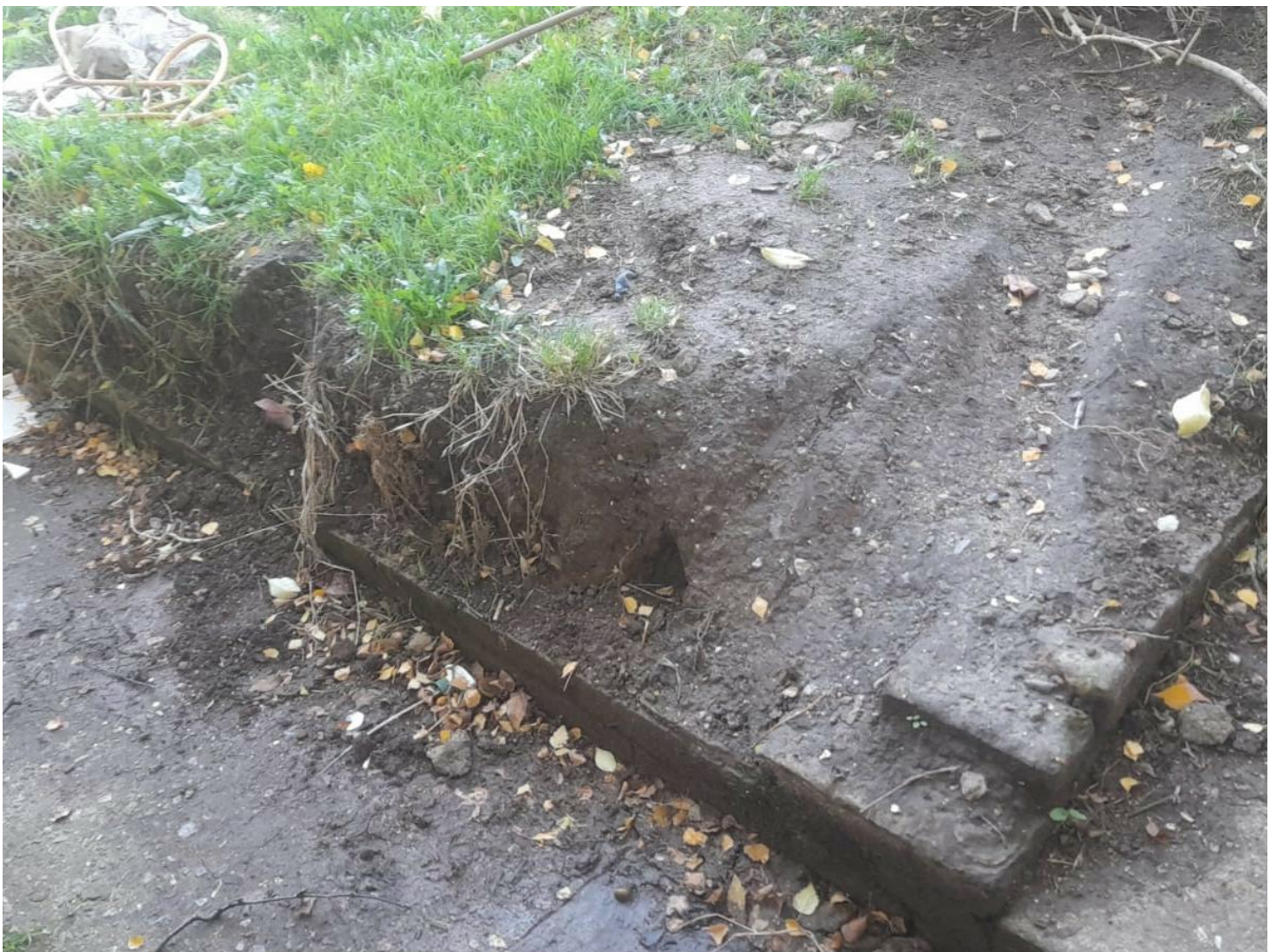
Photograph 06 View of the existing retaining wall which is beginning to fall apart, causing mud to wash over the footpath and steps in wet conditions, making it very slippery and dangerous.
