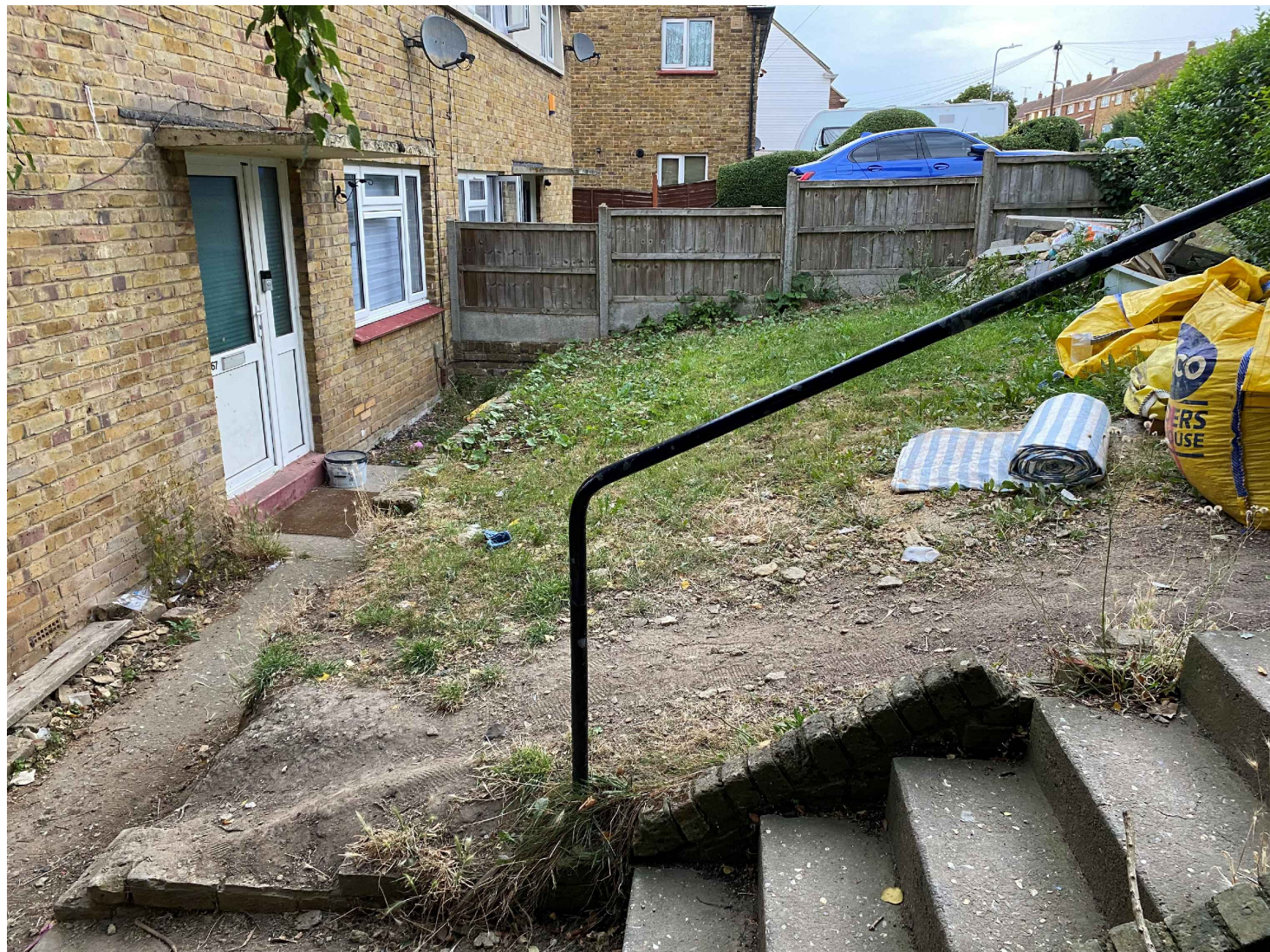
Photograph 02 View of the existing grassed front garden. The slope is unusable due to its steep gradient, and the grass is in very poor condition. The wall to the side of the steps has perished which causes mud to wash over the steps in wet conditions, making it very slippery and dangerous.
