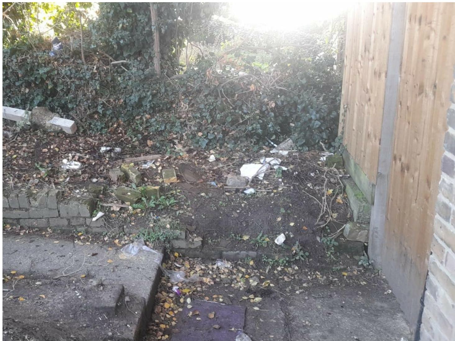
Photograph 05 View facing South-West, showing that the retaining wall to the side of the steps has failed. It can be seen that in wet conditions mud washes across the footpath making it slippery and dangerous.
