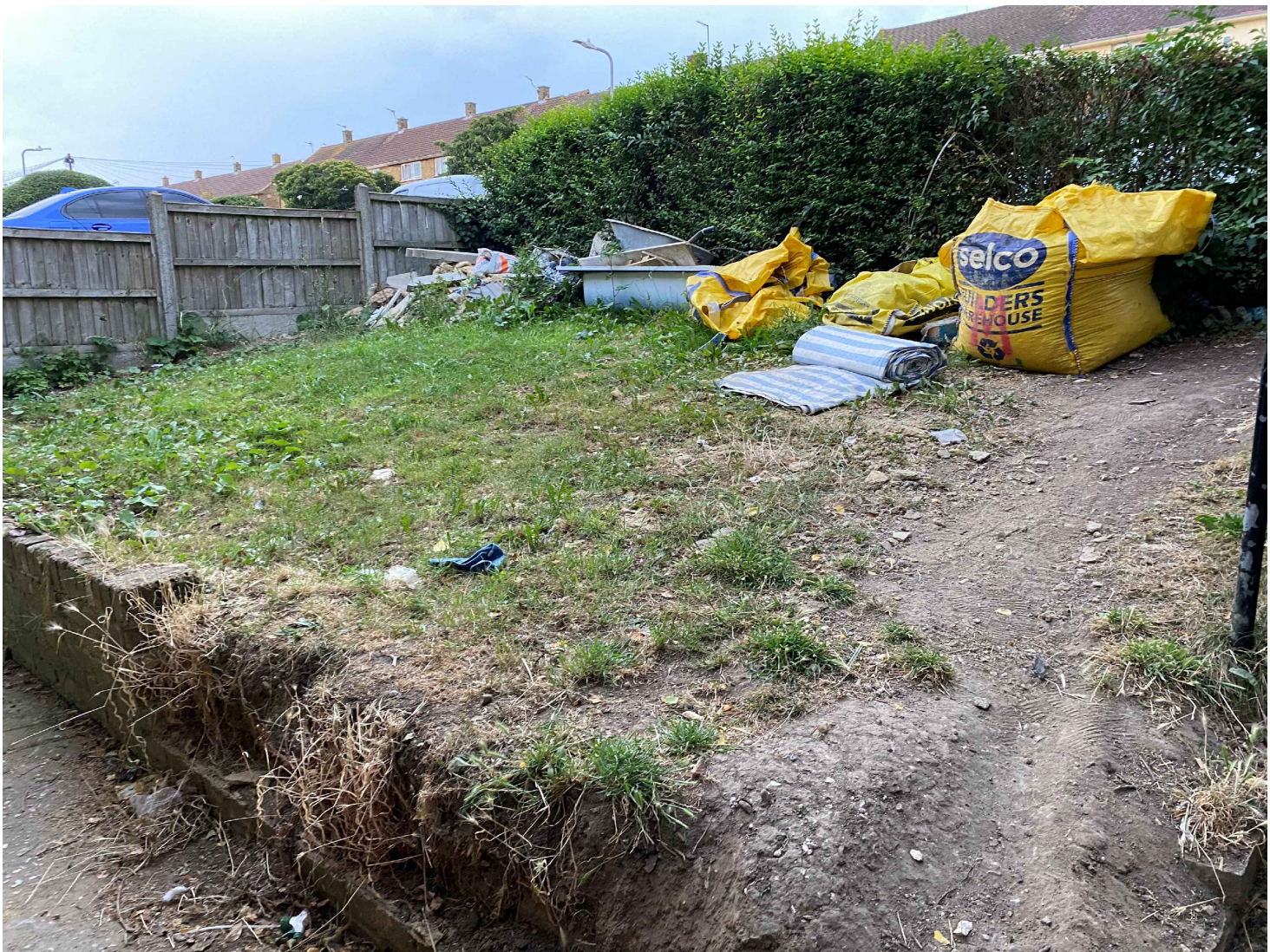
Photograph 03 View of the existing retaining wall which is beginning to fall apart, causing mud to wash over the footpath in wet conditions, making it very slippery and dangerous.
