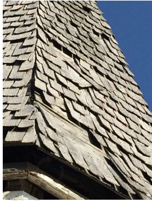
Detail of condition and loss of cedar shingles at St Mary's
