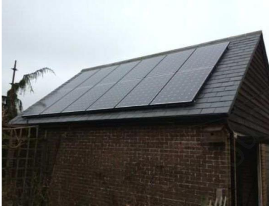
Sample of solar panels
