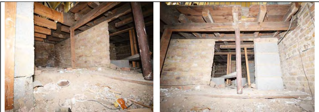
Plate 55: Two access hatched leading from the room under the northeast corner of the nave to the remainder of the floor of the church the later joists and block-work indicate intervention for stability in response to the changing use of the building from the second half of the 20 th century
