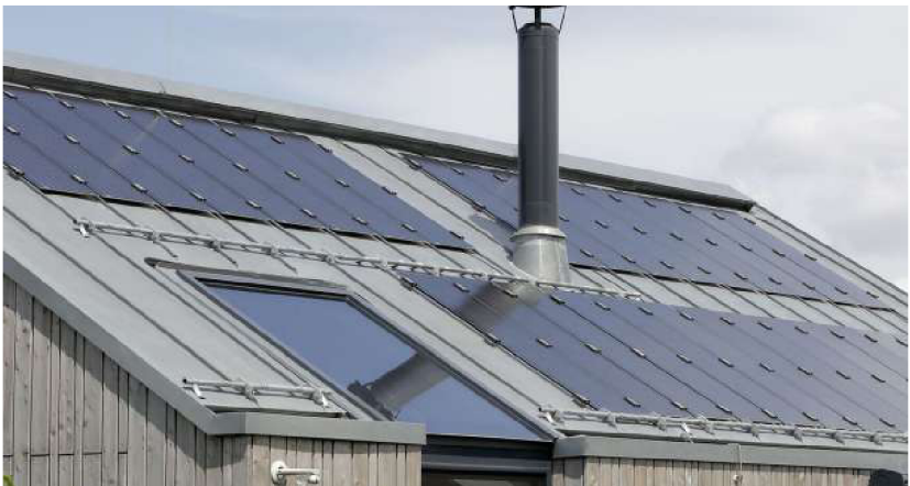
Solar PV cells on Zinc roof
