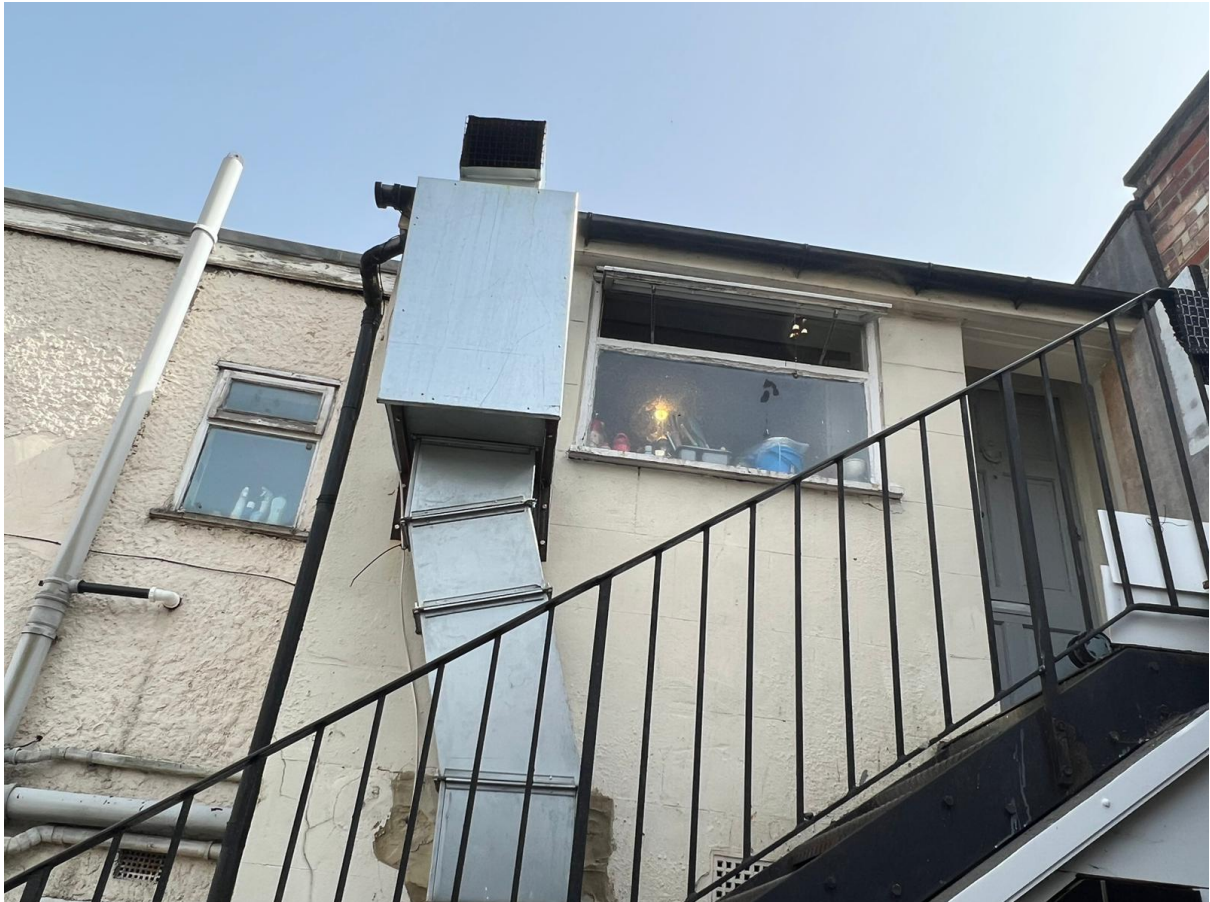
Photograph showing rear of extraction system.
