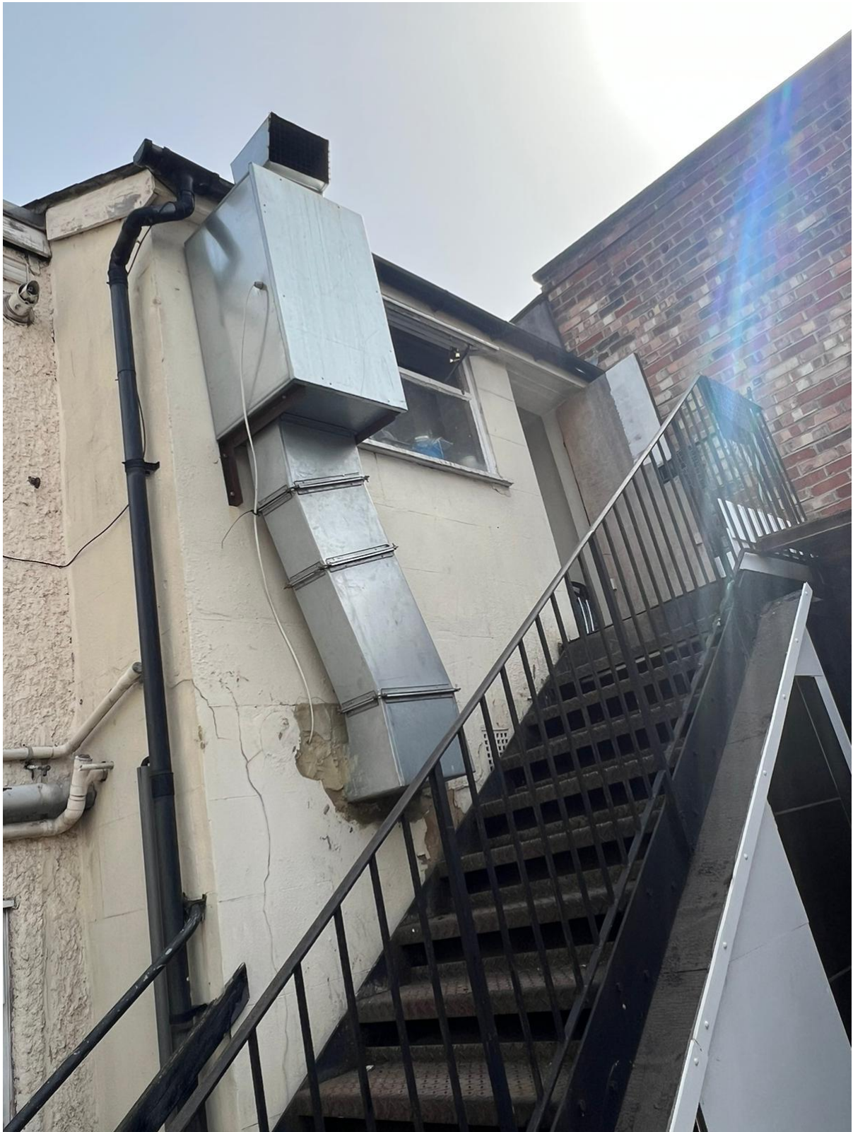
Photograph showing side of extraction system.
