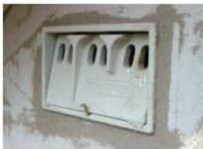
1SP built into a wall
