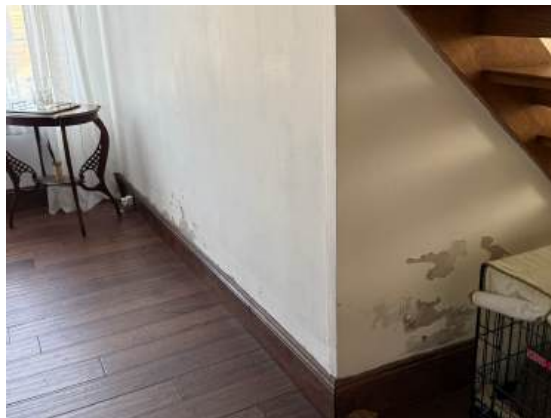
Fig 14 – Damp internal brick walls with cement based plaster finish.
