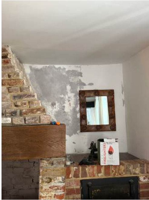
Fig 13 – Damp external walls with cement based plaster finish.
