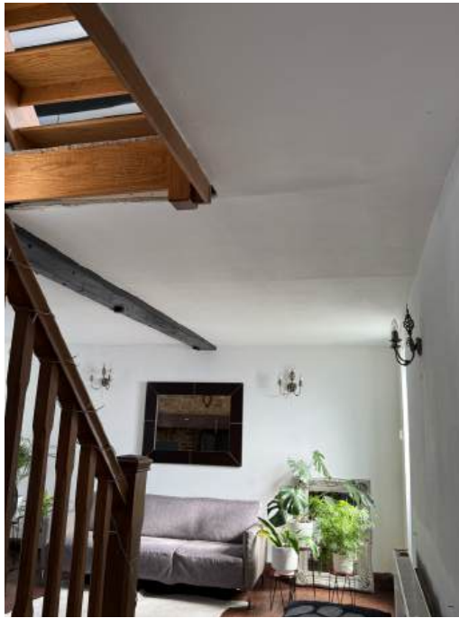
Fig 08 – Ceiling marks indicating location of removed stud wall
