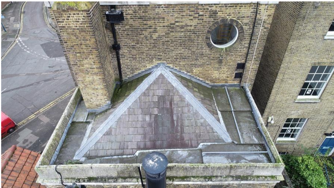
Fig 55 View of the north wall of the east wing and lower bay on its north end showing the later chimneystack in front of the oculus window. Removal of the stack would allow the window to be reopened. Note the cast lead hopperhead.
