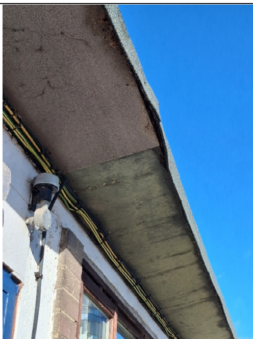
Plate 15. Lifted felt roofing on eastern side of building.
