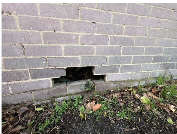
Plate 13. Hole in concrete wall giving access between woodland in west of site and other areas of the site.
