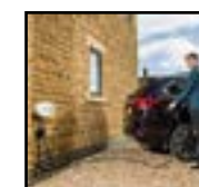
Car Charging Point in Car Port
