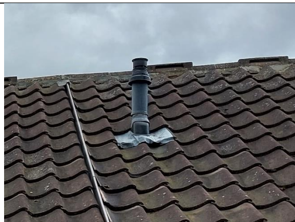
Image 18: gap under the lead flashing on apartment 23.
