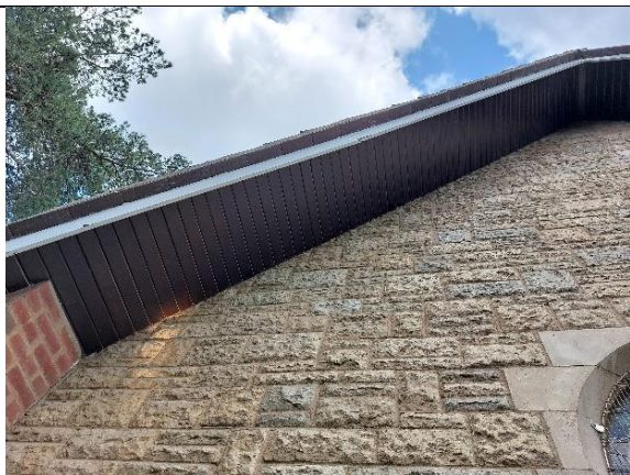
Image 11: gaps between soffit and wall on the chapel.
