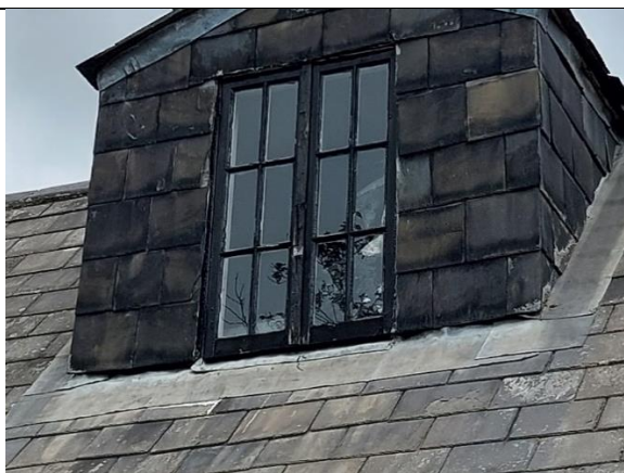
Image 15: gaps under dormer slates on Chaplain's house.
