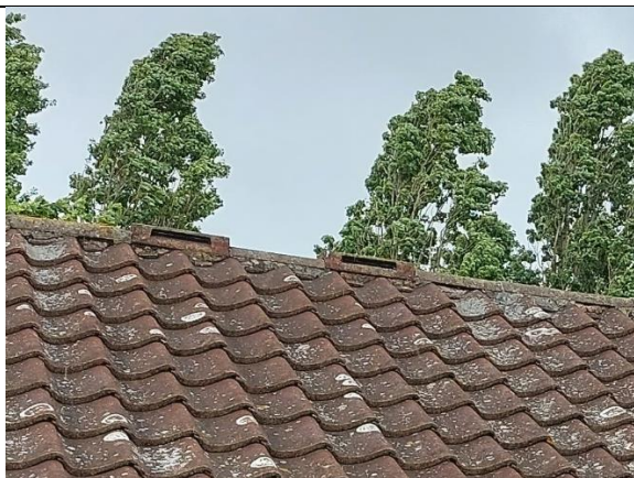
Image 17: gaps under the ridge tiles on apartment 20.
