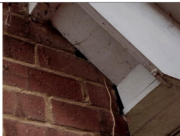
Image 16: gaps at the gable end of apartment 15.
