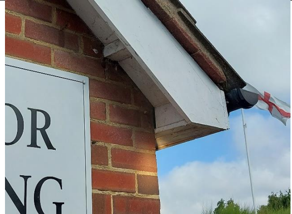
Image eight: gaps in the soffit of apartment 1.
