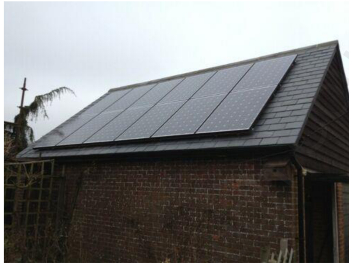
SAMPLE OF SOLAR PANELS
