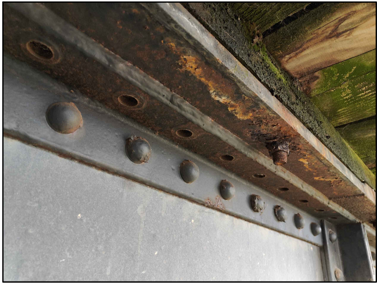
PHOTO 3 - SUPPORTING STEELS WITH TIMBERS IN POOR CONDITION
