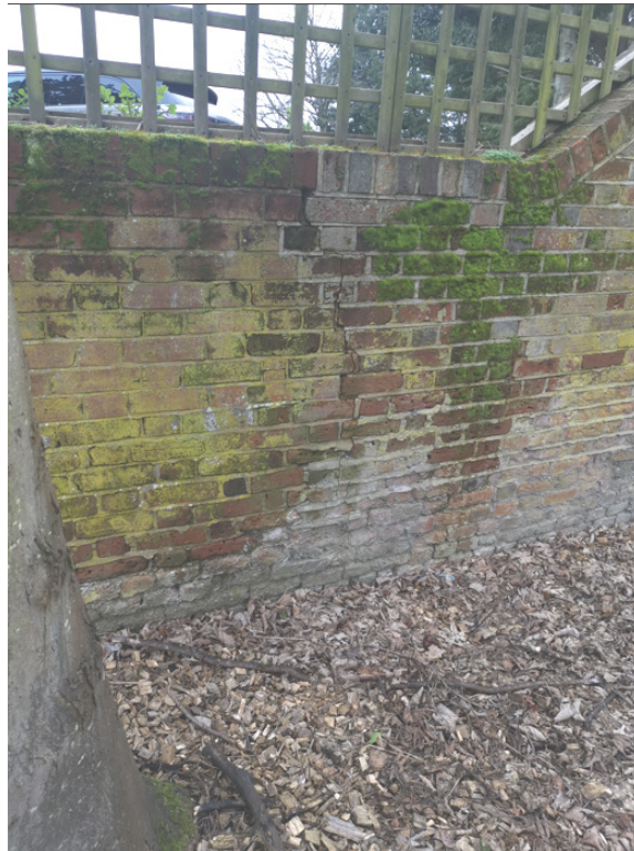
P004 – number 4 repair required
