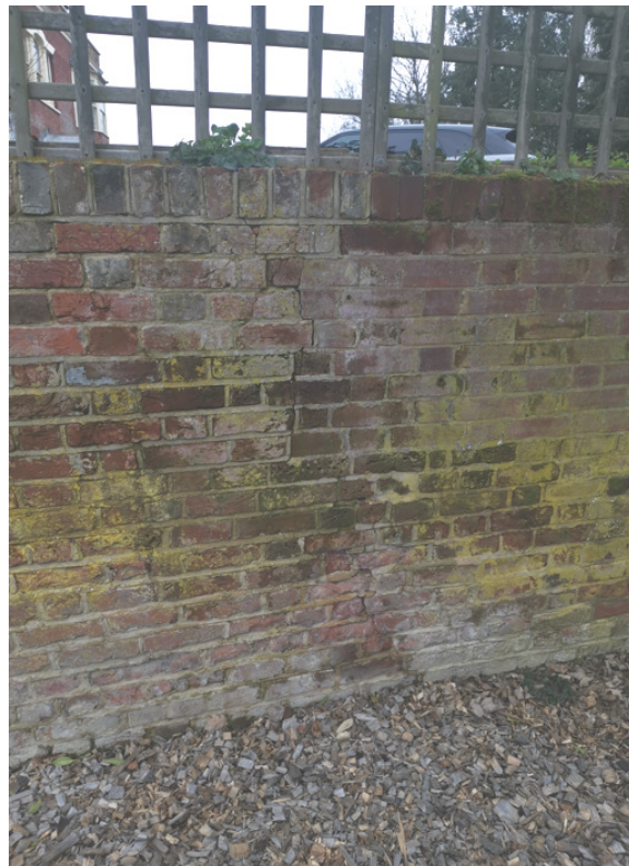
P003 – number 3 repair required
