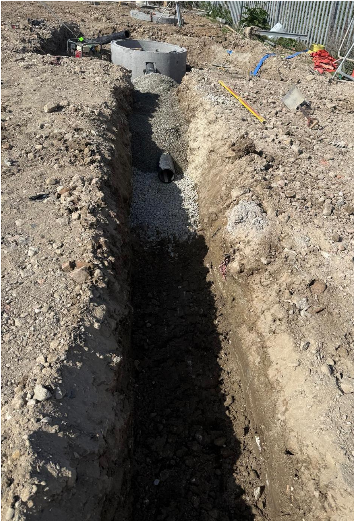
Drainage run to Hydrobrake and Interceptor.
