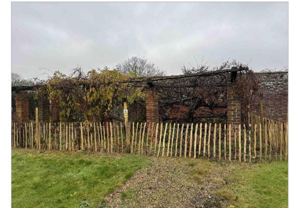
3. VIEW SHOWING PLANTING & COLLAPSED ROOF
