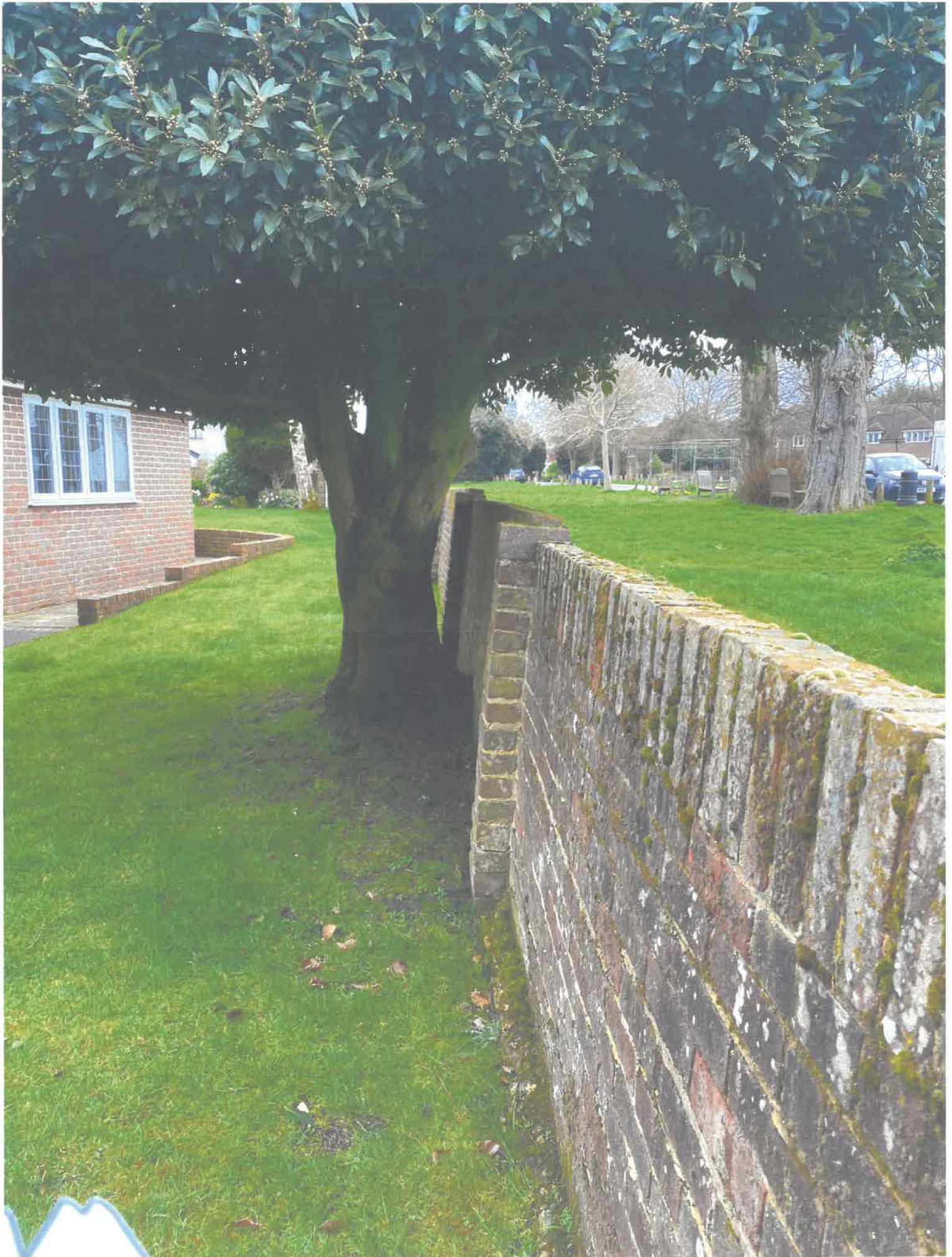
Bowing of wall outwards,
