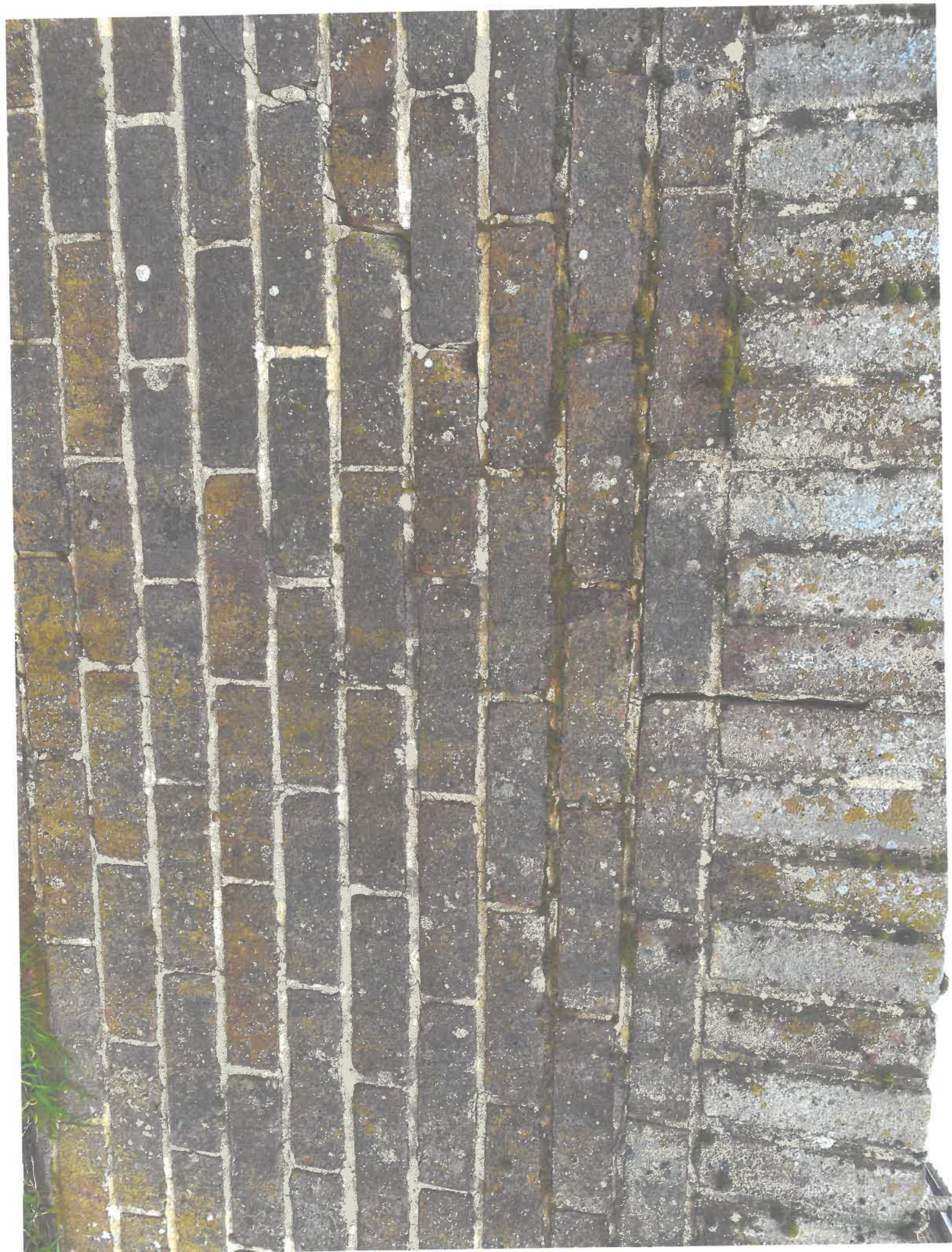
Damage to wall & bricks
