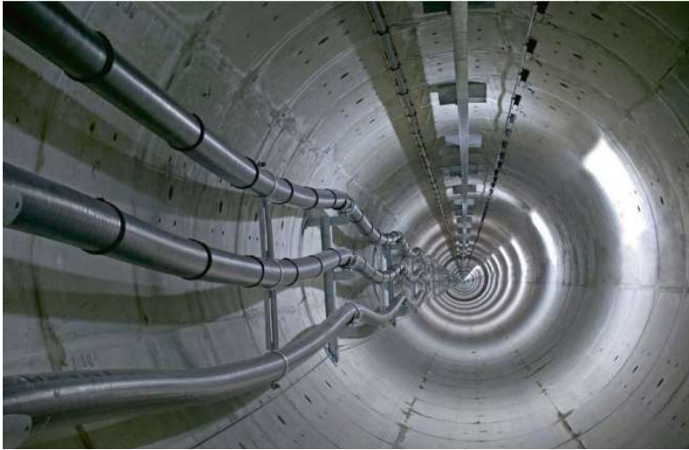
Photo 1 XLPE Cables installed in a deep bore tunnel
