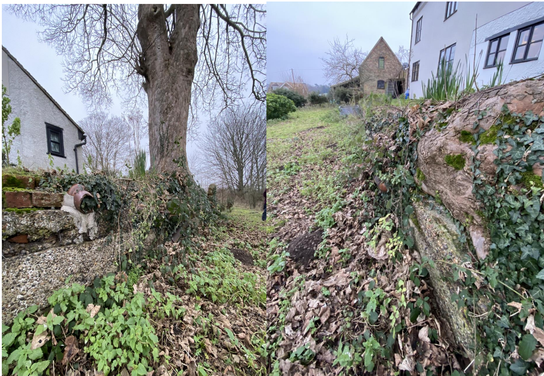
Fig.2; Sycamore T1. Large structural roots at the base of the bole having entirely displaced capping. Rebuilding wall to this level would require severance or trimming of these roots leading to structural instability and large wounds as entry points for decay
