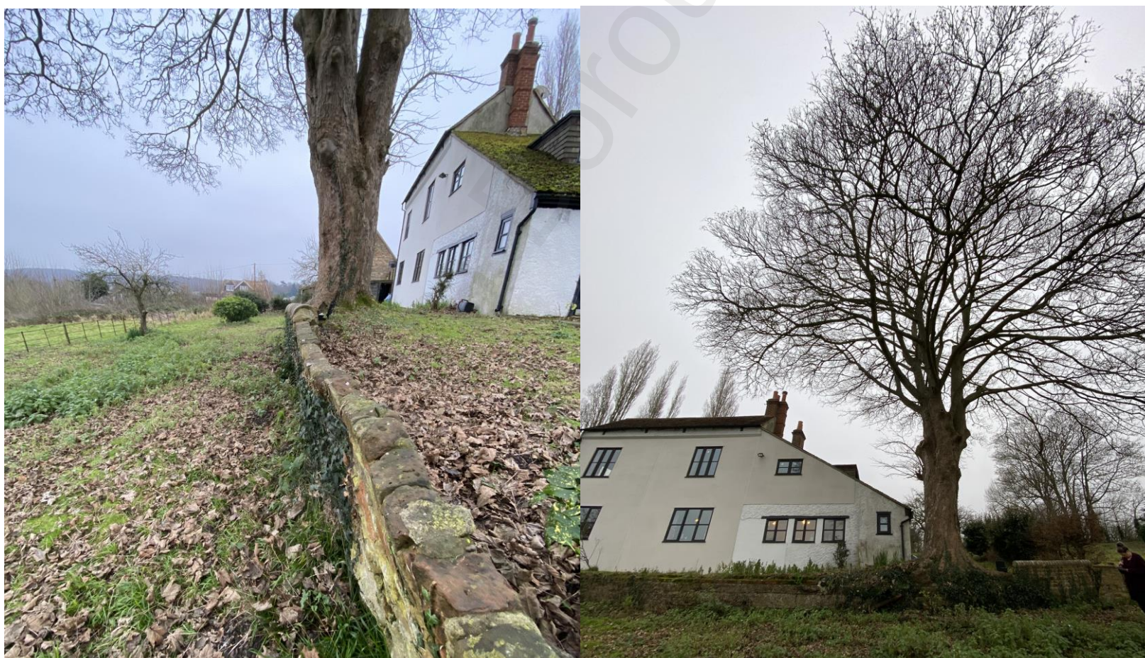
Figure 1; Sycamore T1 growing against the retaining wall. Note the displacement and bulging of the wall and displacement of the capping bricks.
