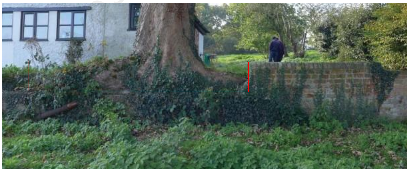
Fig.3; Stem base of T1 against retaining wall of terrace. Red line details sections of root or bole which have grown through or over the wall.
