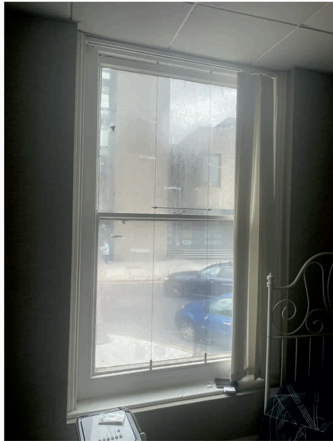
ROOM 2 - Original sash window in good order to be made good. Note there are no window bars and no sign that original bars have been removed, also front wall built out with internal stud work (find out why?).
