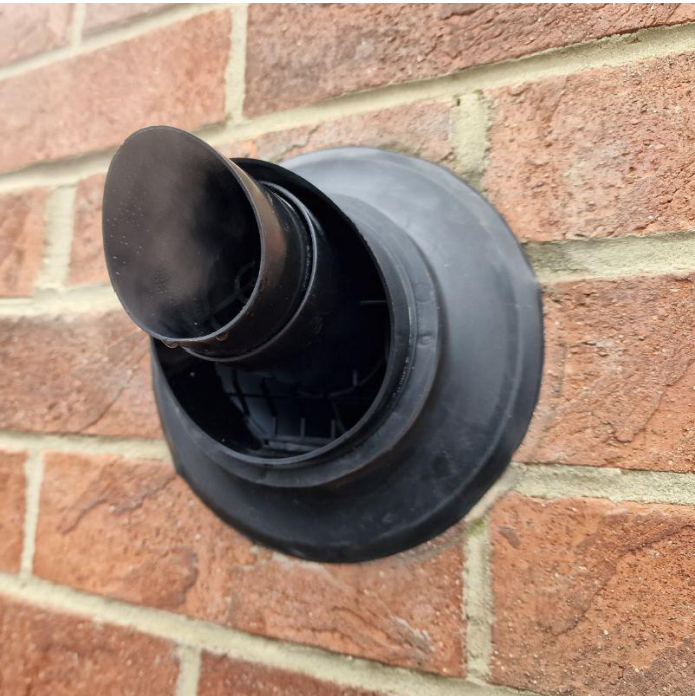
Indicative AGA & Boiler Flues
