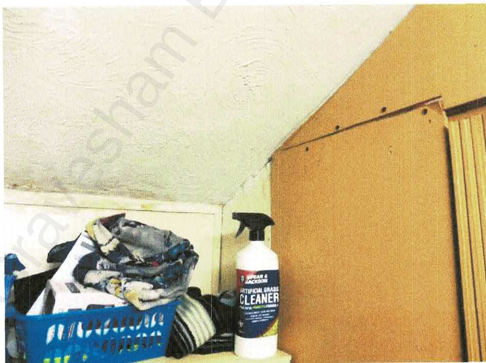
Damp ingress at eaves on South Wall
