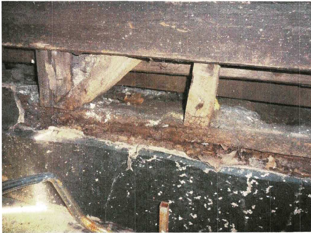
Deterioration of plate and studs to timber frame on South Elevation
