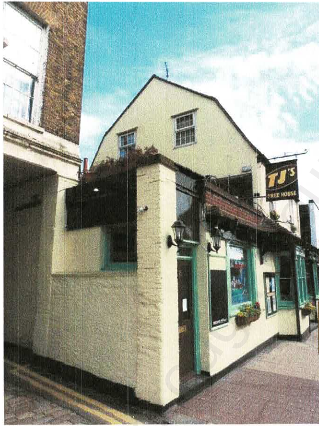
Front Elevation with out of vertical brick pier on Northwest corner
