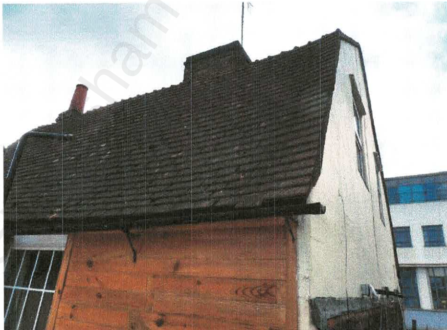
Main roof (Showing sag to slope and distortion at eaves)
