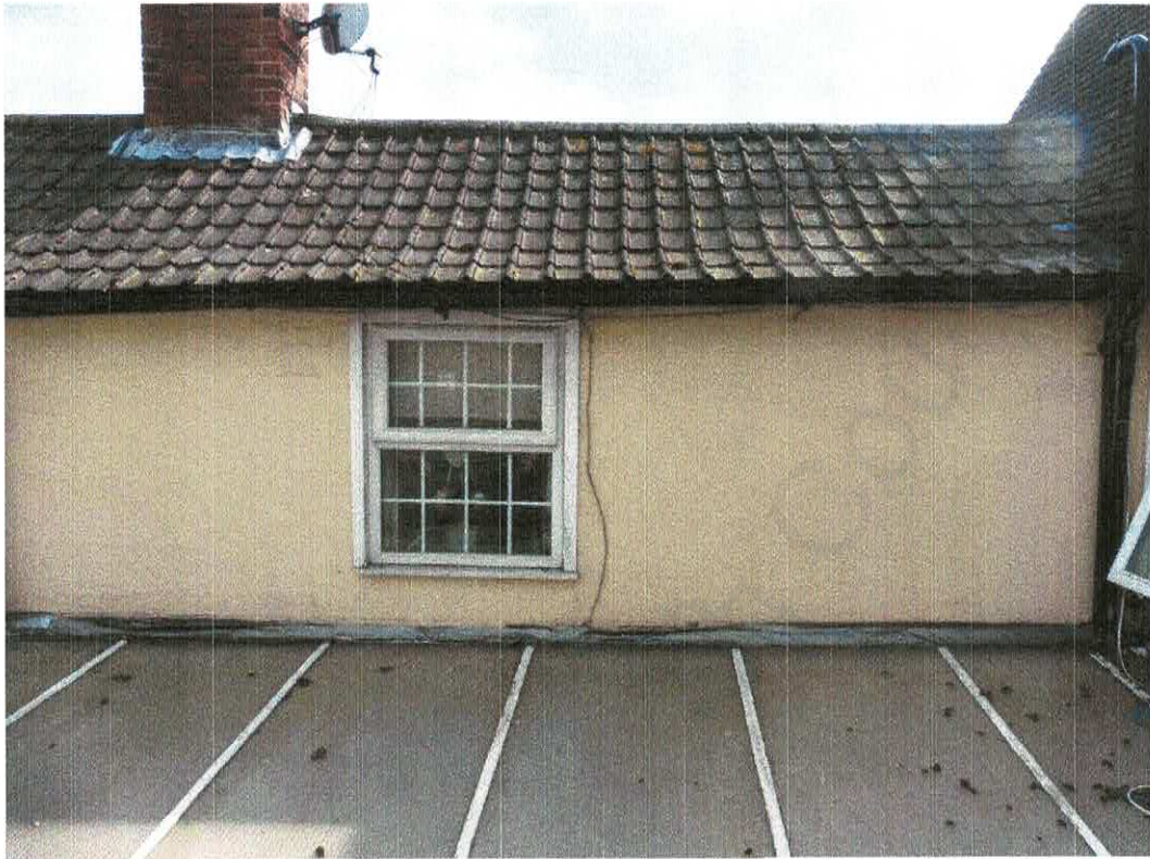
Roof to rear addition (Showing sag to roof and distortion of eaves)
