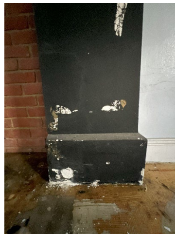
Close up of wear and tear to surround.
