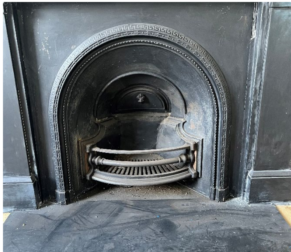
Minor damage where insert abuts the surround.
