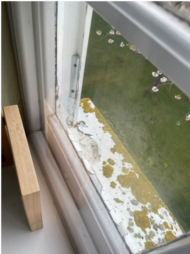
Figure 6 Example of rot and damage to the windows
