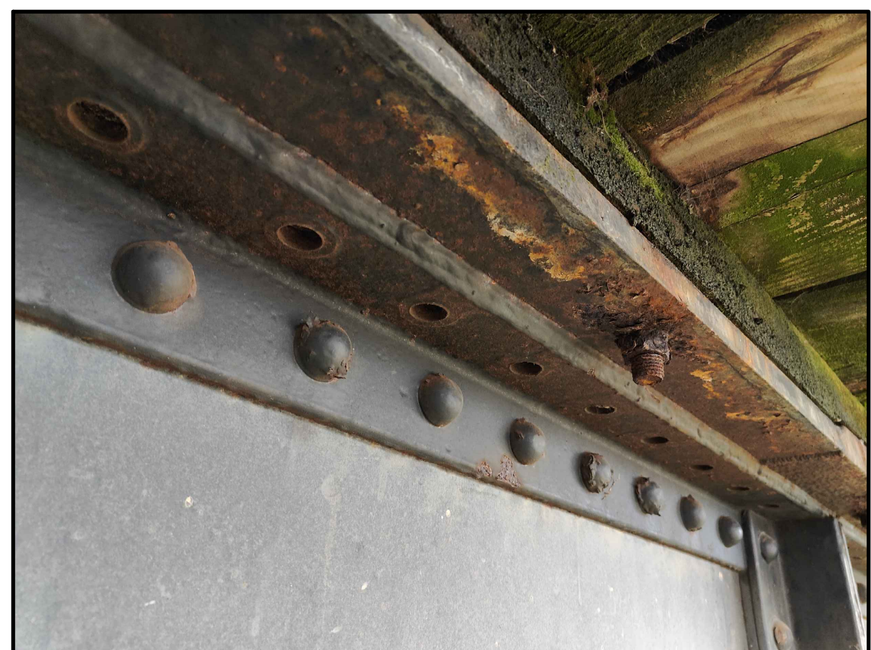
PHOTO 3 - SUPPORTING STEELS WITH TIMBERS IN POOR CONDITION
