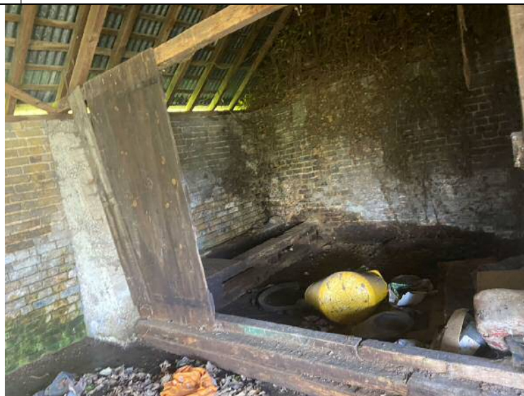
Photo 4: Staining on barn floor from historic usage.
