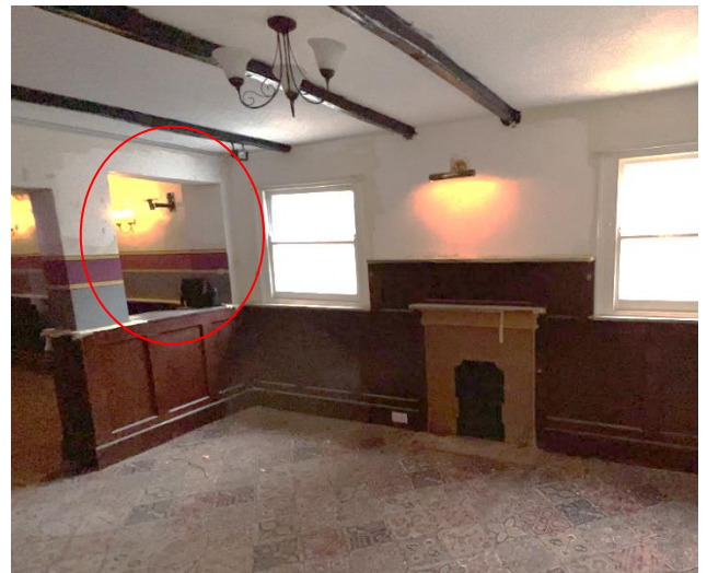
Figure 13. 1980s Rear extension with window aperture ringed in red.
