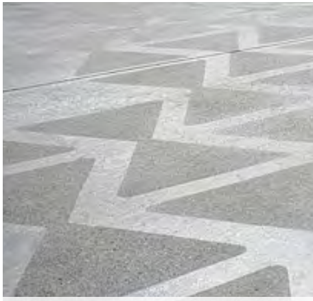
Sand blasted surface
