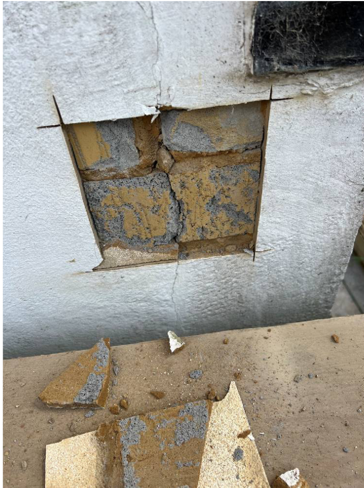
Plate 2 – Cracking to Render and Through Thermalite Blocks
