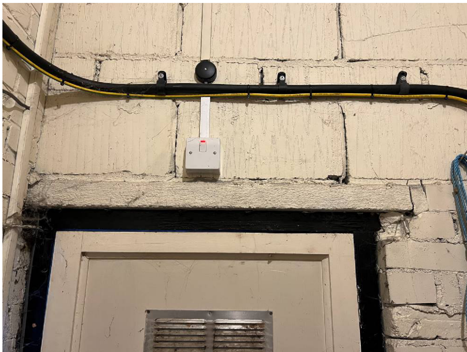
Plate 3 – Poor Lintel Bearing to Boiler Room Door
