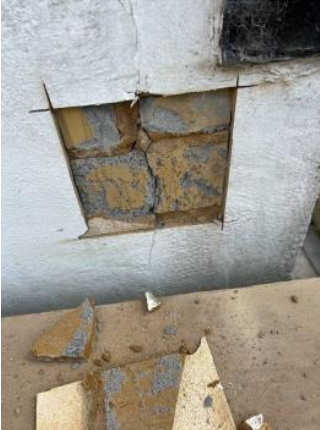
Inspection hole removing render to expose cracked blockwork and mortar joints behind.
