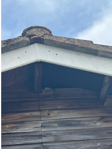
Picture 2: Showing another hole under the end wall allowing for roosting bats to access the roof to roost.
