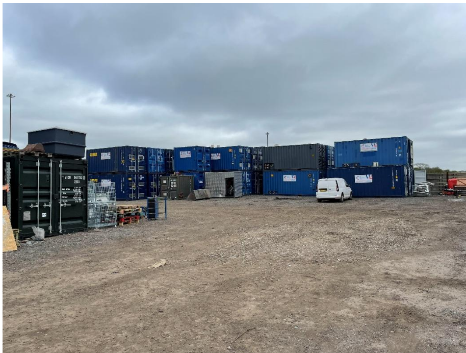
Photograph 3.2 – Storage of the mobile boiler plant rooms on site
