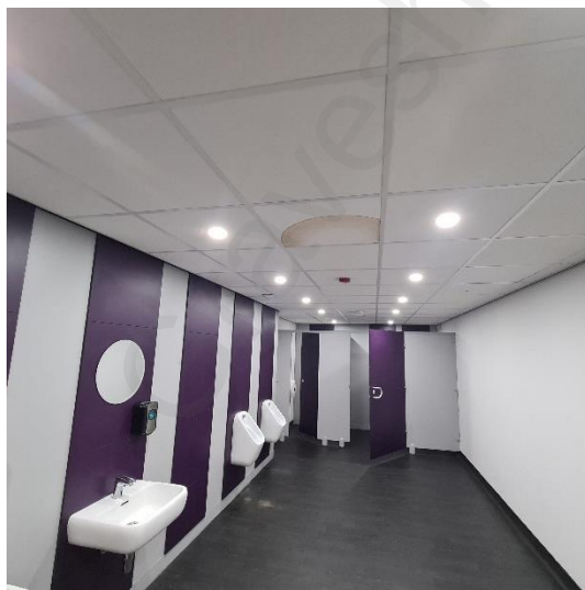
Figure 14: Evidence of water damage to dry change ceiling
