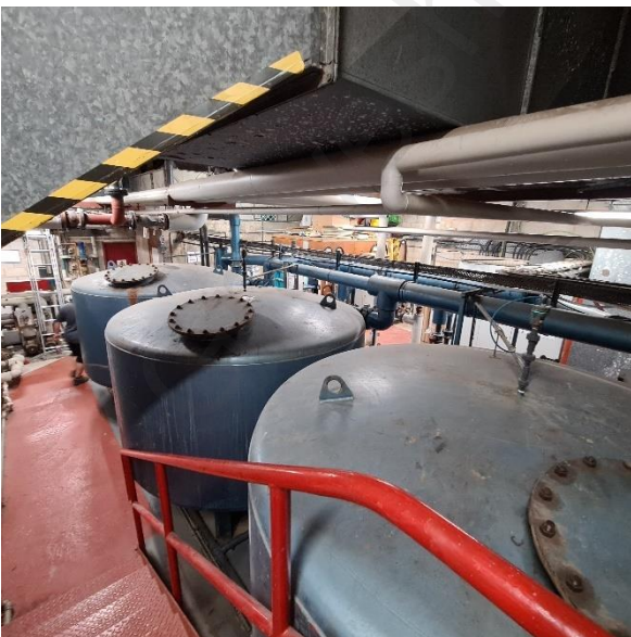
Figure 50: Pool plant room
