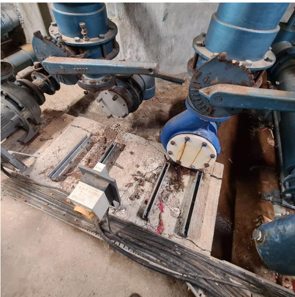
Figure 62: Undercroft damaged concrete plinths
