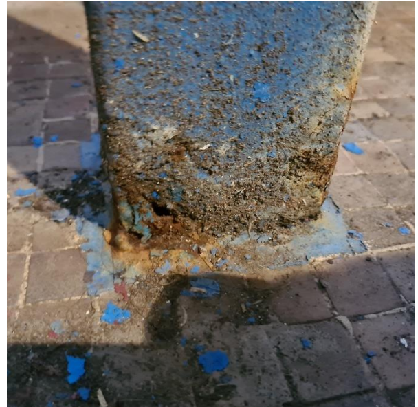
Figure 47: Corroded flume tower steelwork (3)
