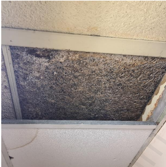
Figure 12: Exposed wood fibre soffit in cleaners cupboard
