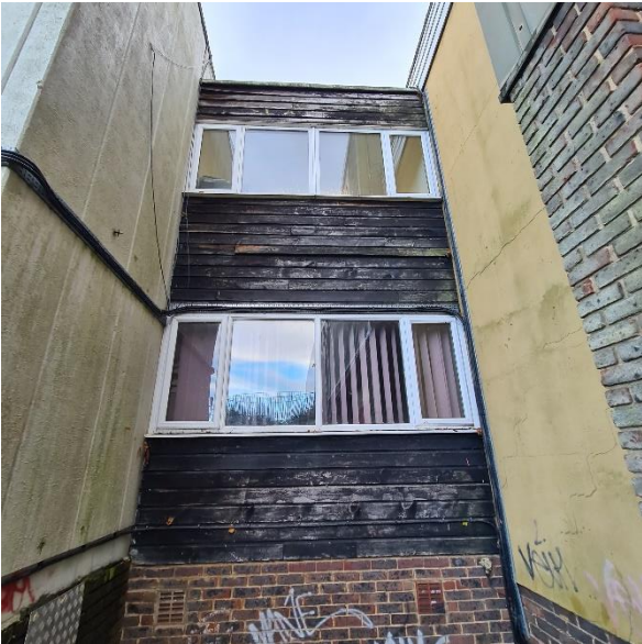
Figure 75: East elevation of squash courts with cracked render and damaged timber
