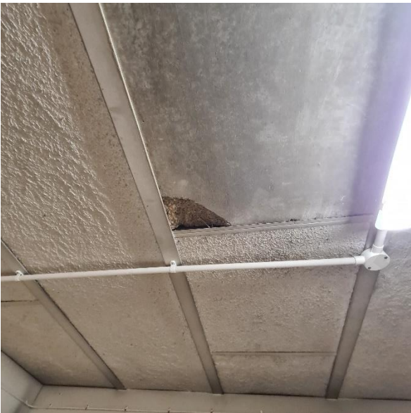
Figure 18: Damage to exposed wood fibre soffit to sports changing rooms (1)
