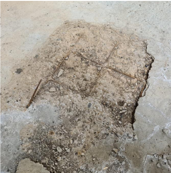
Figure 60: Damaged undercroft concrete base slab (3)
