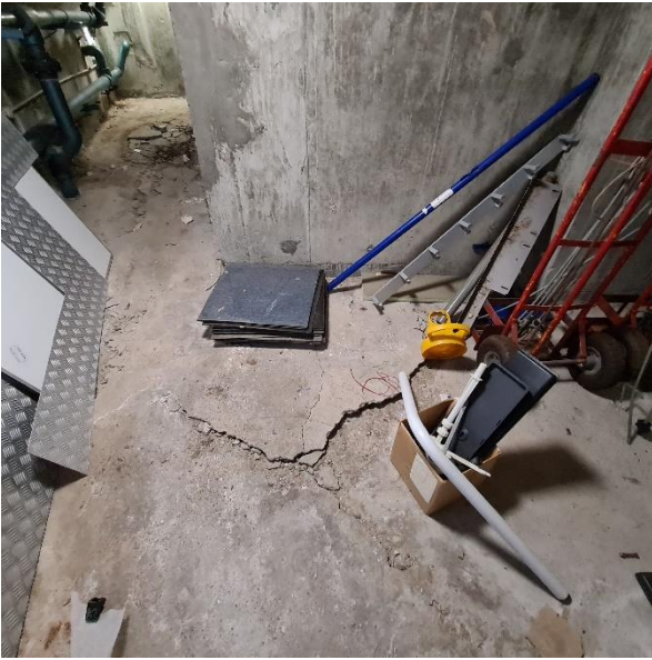
Figure 58: Damaged undercroft concrete base slab (1)
