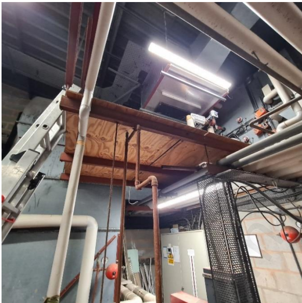
Figure 54: Corroded secondary steelwork in pool plant room
