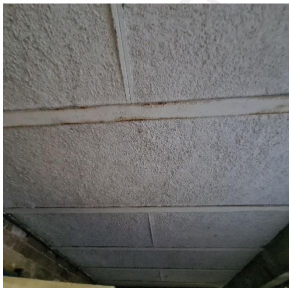
Figure 20: Corrosion to steel rib of sports changing room roof slab soffit
