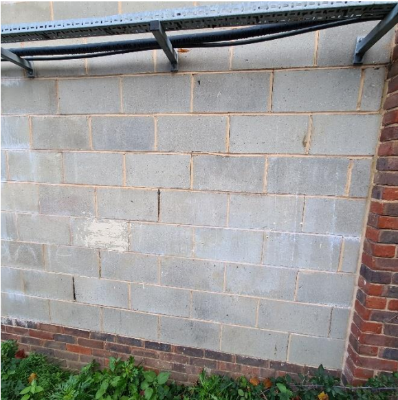
Figure 81: Damaged blockwork to west elevation of pool hall and plant room
