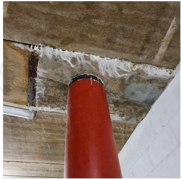
Figure 49: Corrosion to capping structure to pool store
