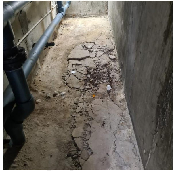
Figure 59: Damaged undercroft concrete base slab (2)
