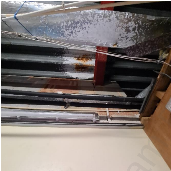
Figure 66: Corroded steelwork adjacent to first floor spa
