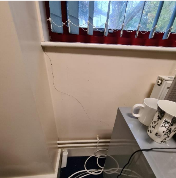
Figure 16: Cracking to internal plaster finish of office external wall
