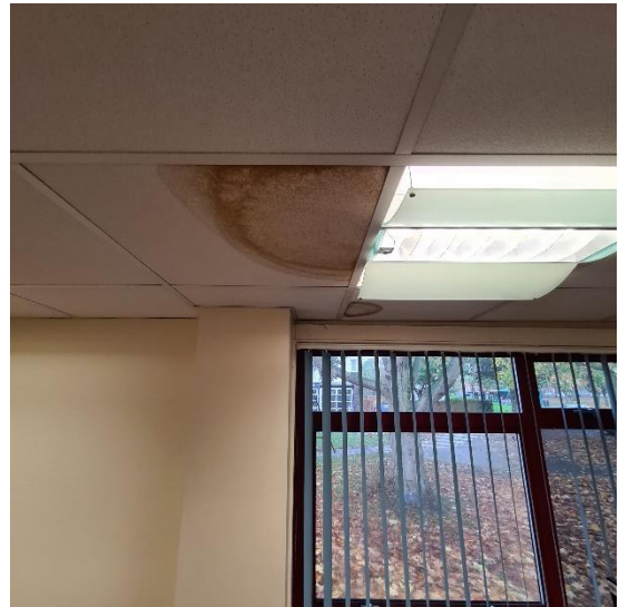
Figure 15: Evidence of water damage to office ceiling
