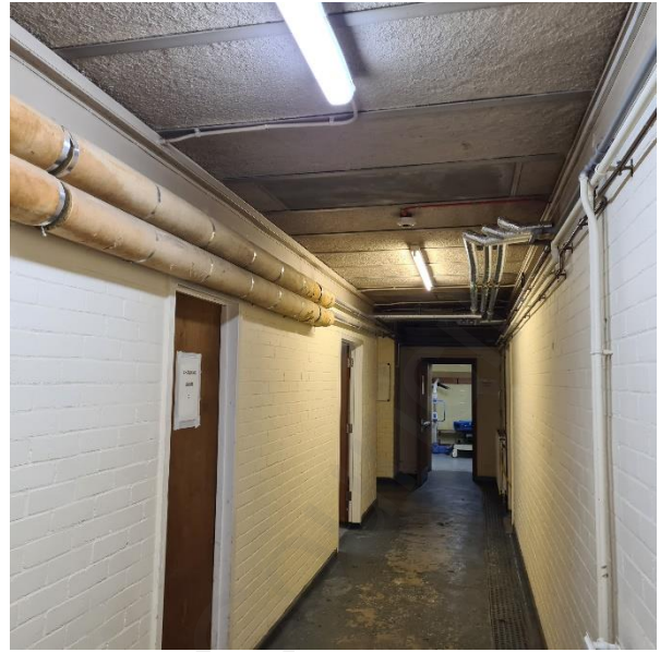
Figure 17: Exposed roof slab soffit to sports changing rooms
