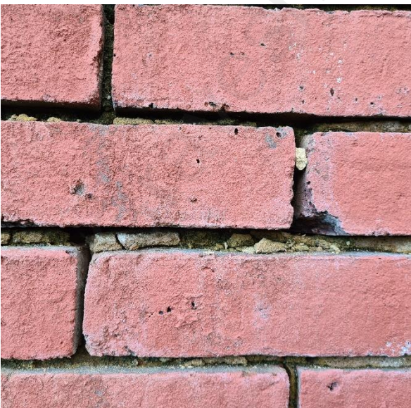
Figure 79: Mortar bed joint loss to squash court external brickwork (2)
