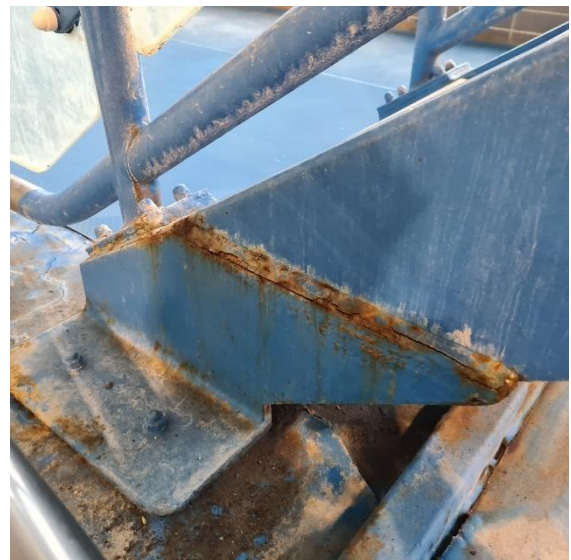
Figure 45: Corroded flume tower steelwork (1)
