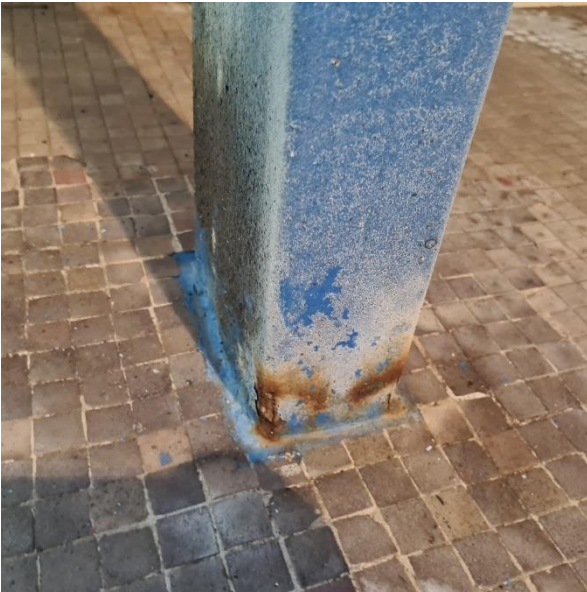
Figure 46: Corroded flume tower steelwork (2)
