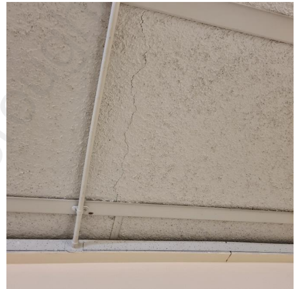
Figure 19: Damage to exposed wood fibre soffit to sports changing rooms (2)
