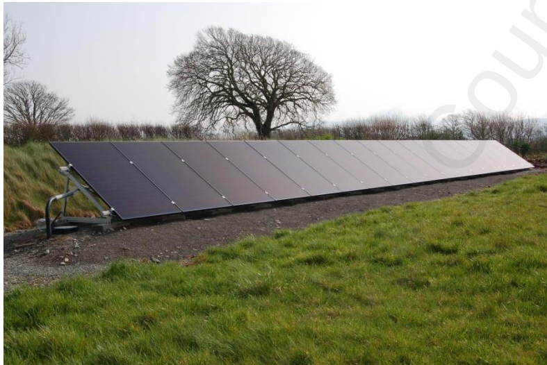
Figure 2. Typical array using Renusol Trisole TS+ mounting equipment
